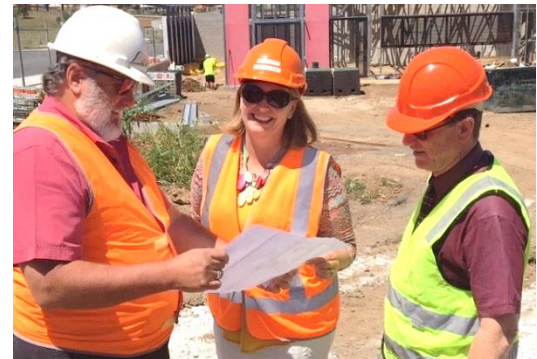
Lawrie Bertoldi, Deidre Young and Gerry Conway review the site plan for Stage 2 of McAuley College.
